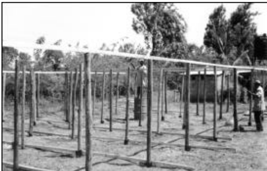
Construction progresses in late winter and early spring of 2003 on the expanded nursery at the Moshi Mpingo Plot. Approximately 7500 sq. ft. is being covered by bamboo slats laid on this framework of posts and timbers to provide shade for new tree seedlings.
